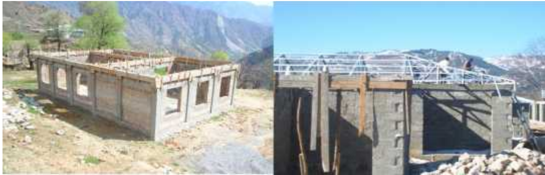
Figure 5 & 6: ERRA-NESPAK Construction Technique Using Brick (Left) and Concrete Blocks (Right) in the area at a large scale and it became popular even in the subsequent self-made constructions.
