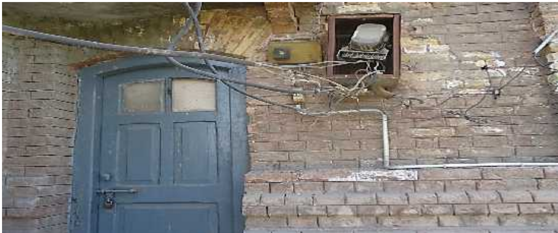
Figure 7. Lack of electric system management
