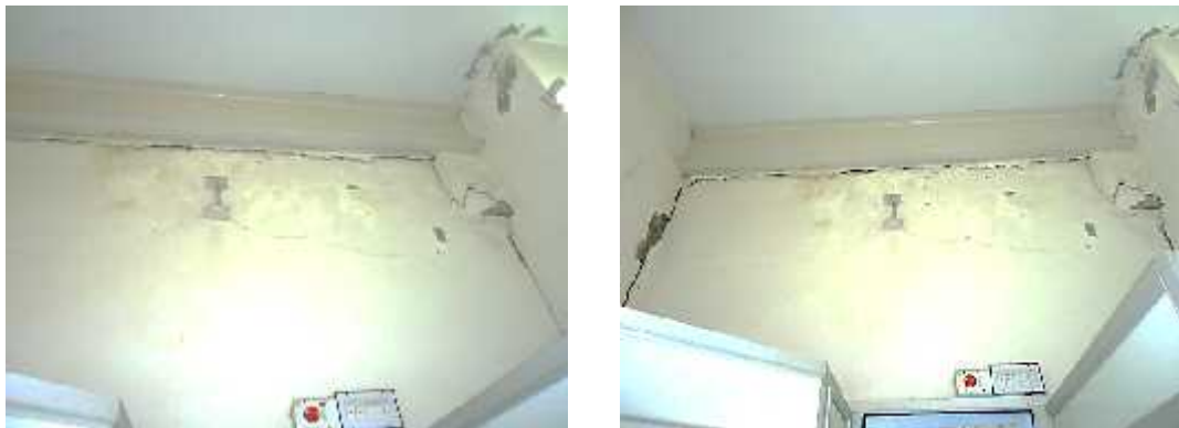
Figure 2. Cracks and seepage in the museum building
